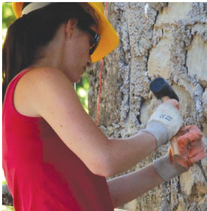
Heather Dowling removing cement from the historic Panagia Vlaherna chapel, Romiri, Zakynthos, Greece. Heather is now working as a heritage interpretive planner.
